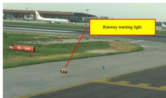
Fig. 6. Runway warning light
